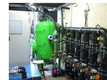
Pump & Treat Anlagen
